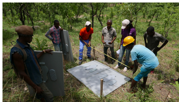
Building of latrines in Anyake Settlement near Adikpo, Photo: Iker Montes-Burgos/Norwegian Church Aid
